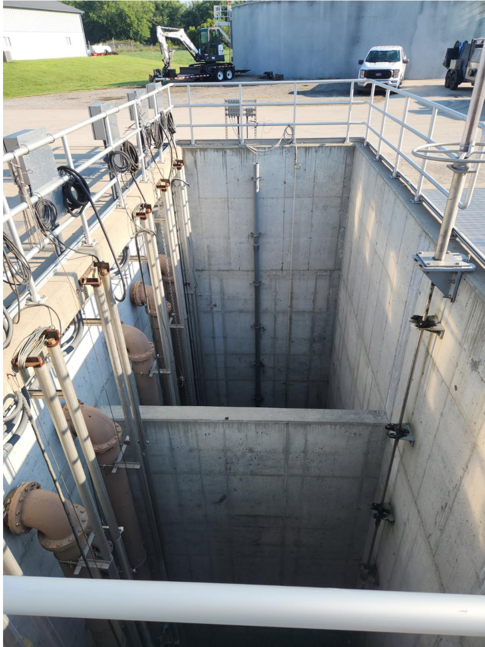
Influent Pump Station – Picture 4
