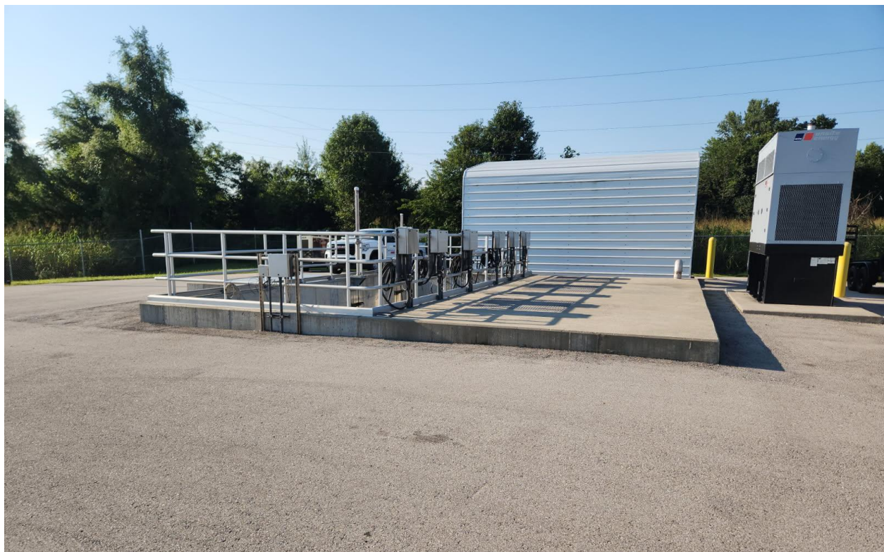
Influent Pump Station – Picture 1
